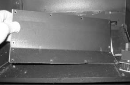
Fan Cover Plate Removed
